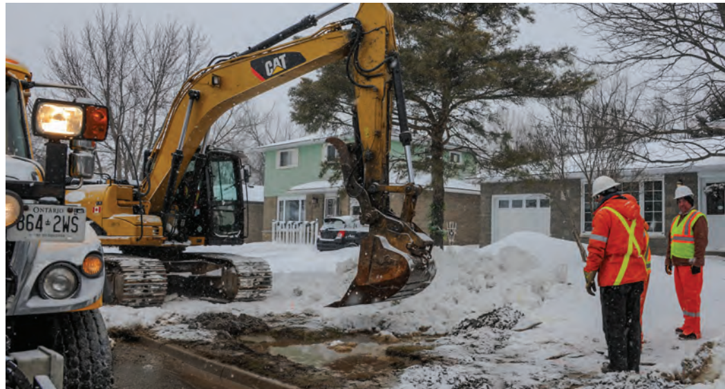
LINE DOWN: Portions of Jelly Street were closed to the public on Wednesday morning (Feb. 27) as Town staff dealt with a water main break. PHOTO: PETER RICHARDSON
